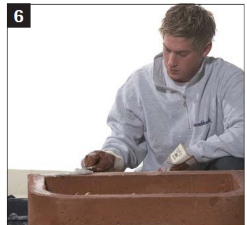
6 Apply mortar on the upper edge of the base and wood storage
